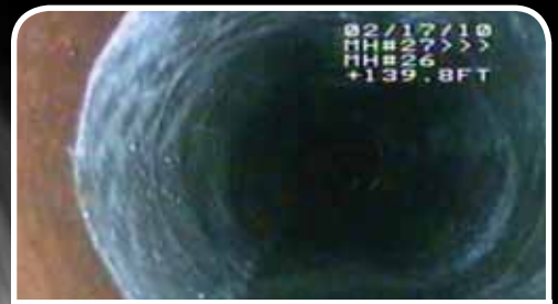
Typical 4' glass resin UV spot repair within 8" vitrified clay sanitary sewer – Milford, Michigan
